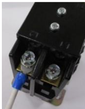
Figure 24: Wiring 220V Contactor
